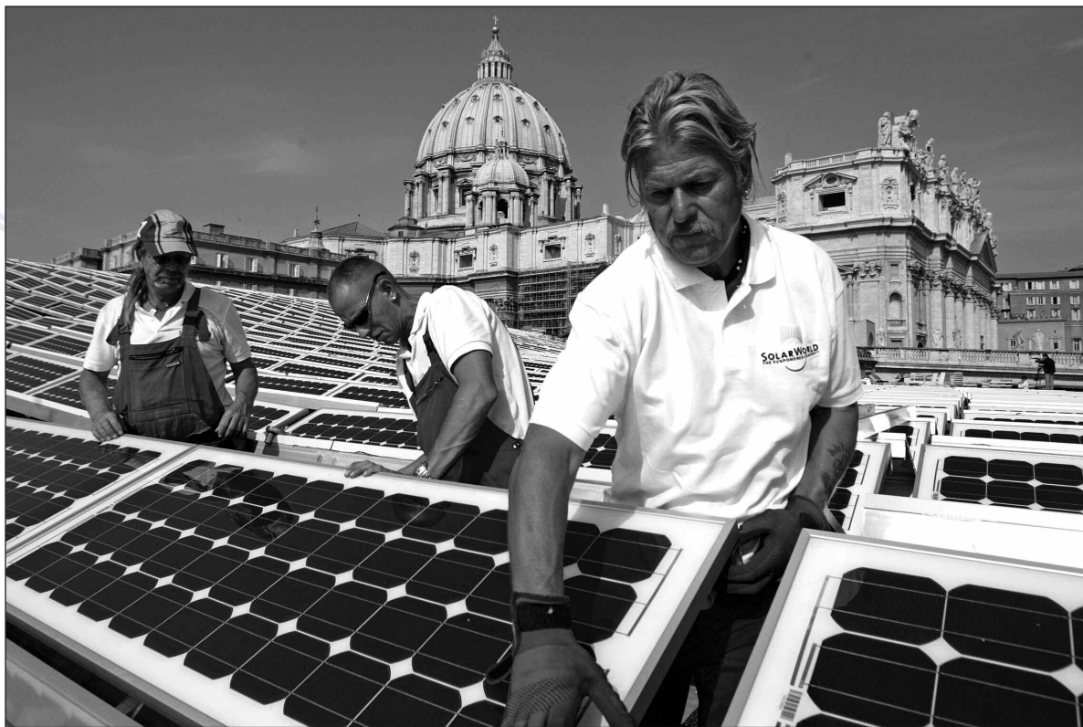
SolarWorld workers install solar panels on the roof of the Paul VI audience hall at the Vatican. The German company donated the modules that will provide the first solar-generated electricity at the Vatican. The solar power system was inaugurated at the Vatican Nov. 26. (CNS photo/Emanuela De Meo, CPP)
